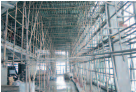
Photo below, top: Rigging used for applying interior finishes. Photo credit: Guido Gilli, Jardine Schindler Hong Kong. Photo below, middle: Technicians install the newest generation of Schindler high-performance elevator drives. Photo credit: Hanspeter Köpfl, Andreas Ryser, Jardine Schindler Hong Kong. Photo below, bottom: The International Commerce Centre rises to become part of Hong Kong's skyline. Photo credit: Sun Hung Kai Properties.
